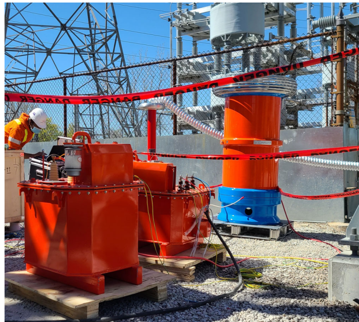
Figure 3. Example of a 70 kV/10A VFRSTS including an isolation transformer, inverter, step-up transformer, HV reactor, and coupling capacitor and used as HV power supply for on-site tests.
